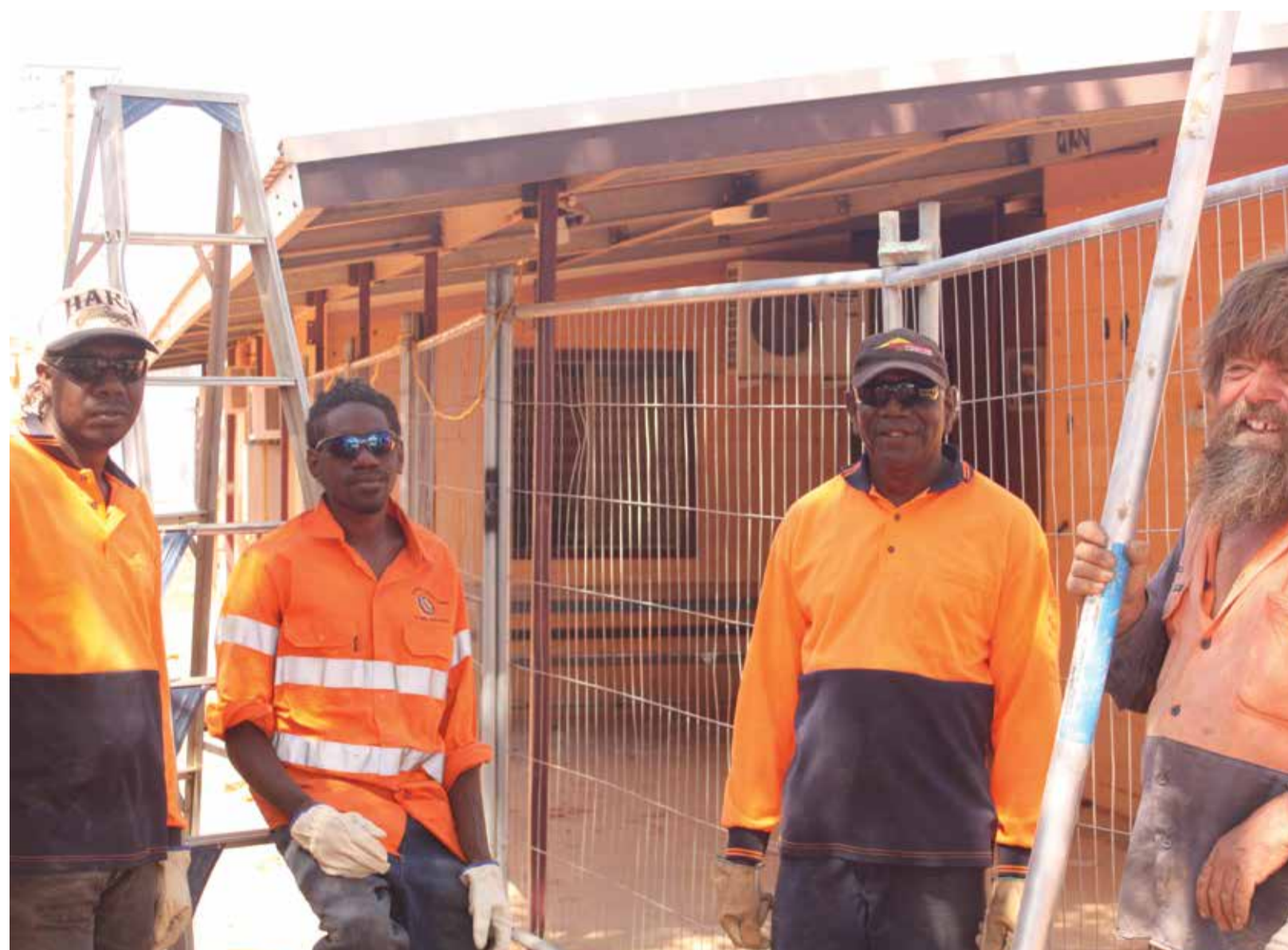
Local men worked with Tangentyere Construction on the Willowra learning centre in 2013. The federal government co-funded this project.
